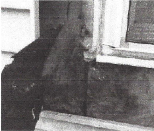
Damage Due to Improper Installation of Windows
